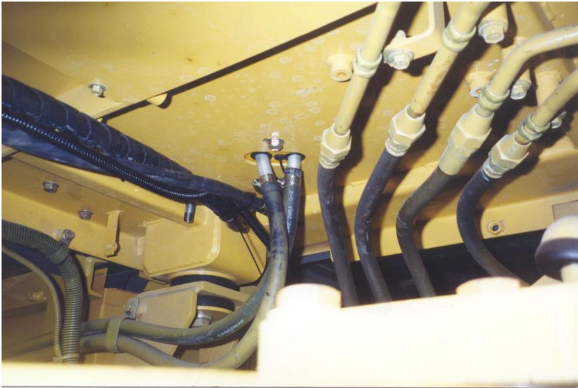
Hoses routed under cab also showing drain extension.
